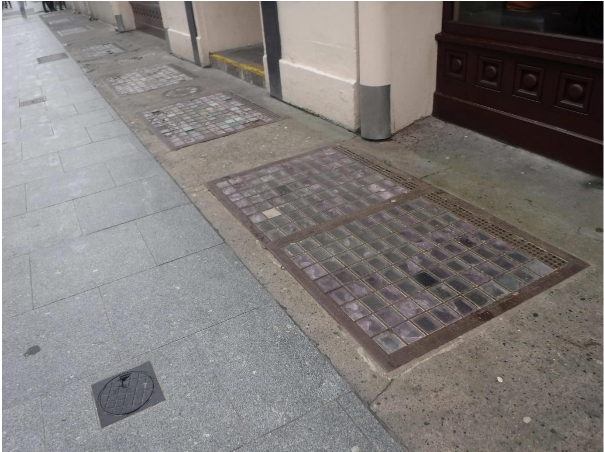
Figure 24 Photograph of cellar lights, Gresham Hotel, Cathal Brugha Street.
